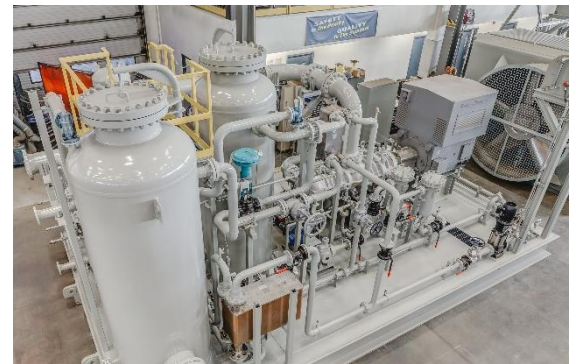
Compression Package | Helium Recovery & Purification
